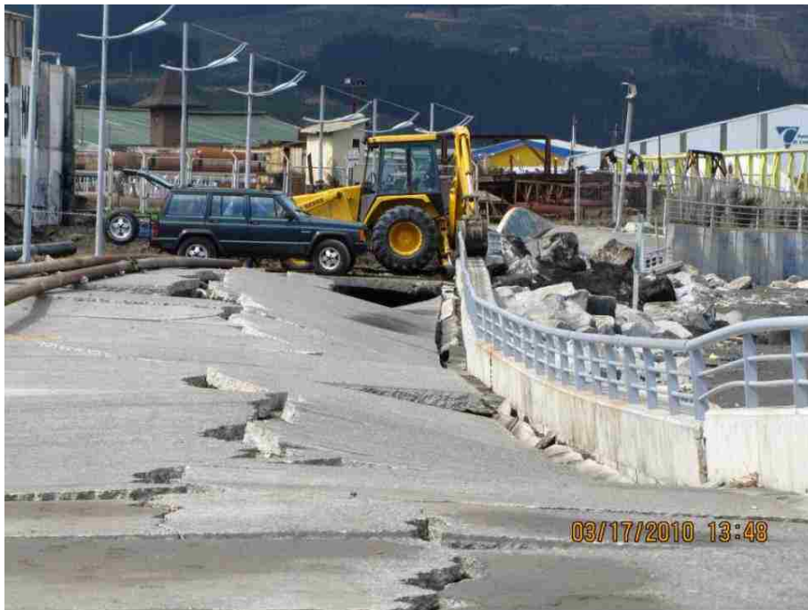
Figure 16. Pavement cracks near Fisherman's (Lo Rojas) pier.
