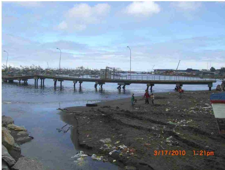
Figure 14. Damages to Lo Rojas pier in Port Coronel due to lateral spreading.
